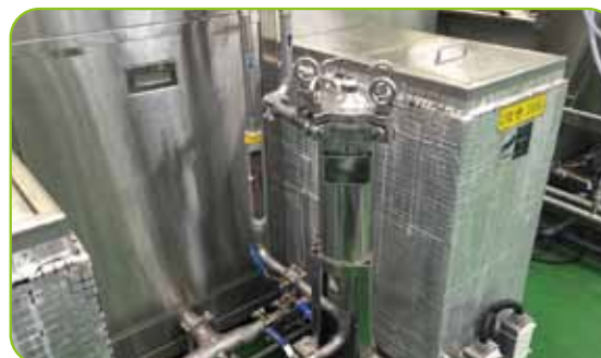
Installation of treatment facilities to increase the number of water cycles (Backflush-type rinsing tanks reduce water consumption and increase wafer cleanliness, supplied water can be recycled and reused)
