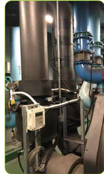
Production equipment improvements (Air compressor and thermal recycling energy conservation improvements)
