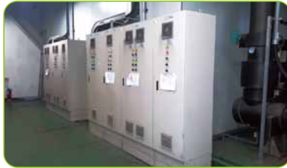
AC system improvements (Chiller system-Cooling tower frequency conversion equipment)
