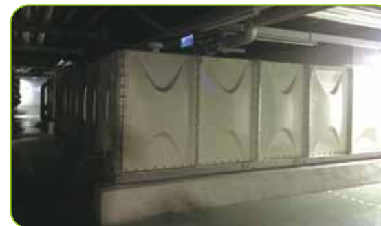
Installation of a water recycling system (Modular water tank recycling system)
