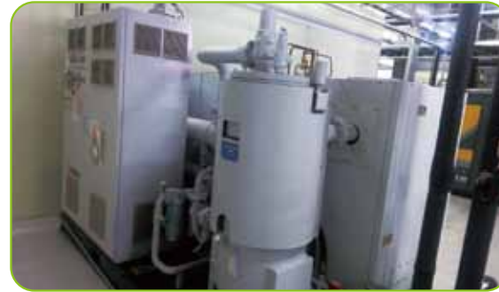
AC system improvements (Installation of VFD air compressors)
