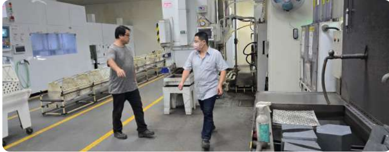
1. Personnel discover a leak in the acid discharge line of the pickling machine and report it to the on-site supervisor.
